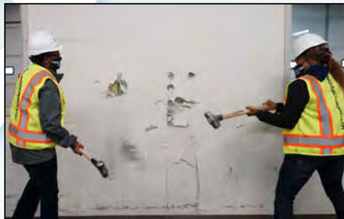
Chancellor Kimberly Beatty (left) and MCC-Penn Valley President Tyjaun Lee did a little demolition work in November 2020 at MCC's new manufacturing training location at 2944 Troost Ave. (It would come to be known as the Advanced Technical Skills Institute.) Although this was a photo op, that wall really did need to come down; renovation was underway. A handful of College leaders also got a tour of the mammoth 101,000-square-foot building from Chief Facilities Officer Jeff Ullmann. The site would house several workforce programs relocating from the Business & Technology campus.
